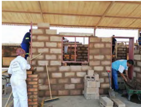
Through an ongoing collaboration with Corobrik, a further 30 people completed a nine-week bricklaying programme, including an all-female cohort of 10 women from the Blackburn community in KwaZulu-Natal (KZN).
