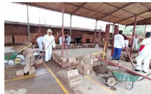
Through an ongoing collaboration with Corobrik, a further 30 people completed a nine-week bricklaying programme, including an all-female cohort of 10 women from the Blackburn community in KwaZulu-Natal (KZN).
